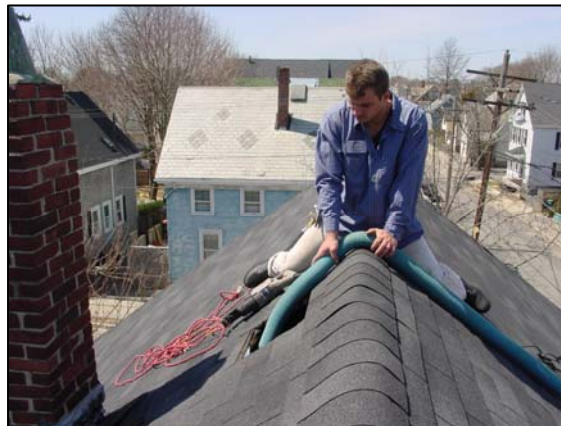
Attic blow through roof in Massachusetts
