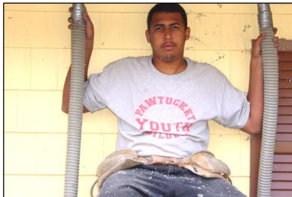
Overhang Blow in Massachusetts
